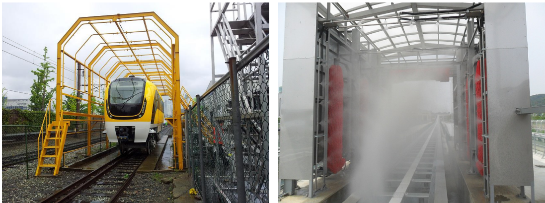
Fig. 3 Waterproof test equipment (in the Factory) and Vehicle washing equipment (in the Depot)
