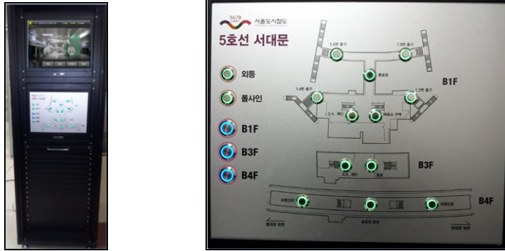
Fig. 3 Manual control panel
