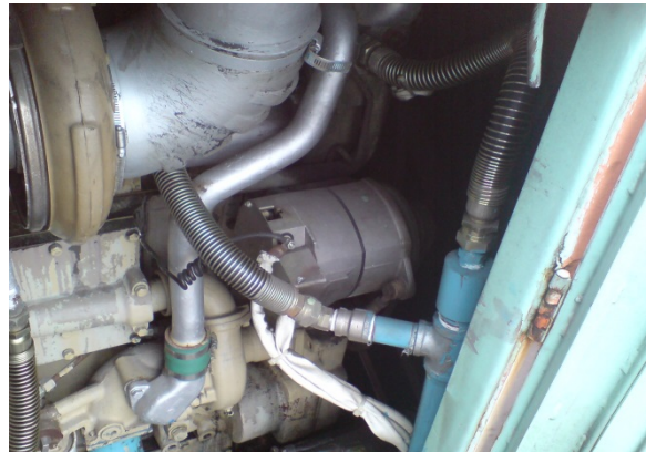
(d) Auxiliary power generator in shunting locomotive
