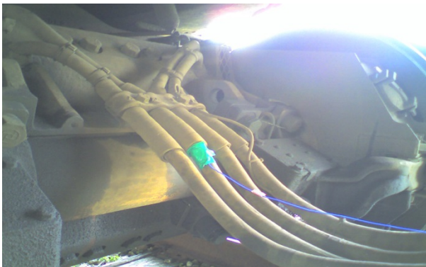
(a) Power cables
