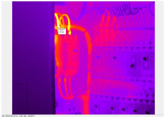
(c) Hot spot on a circuit breaker
